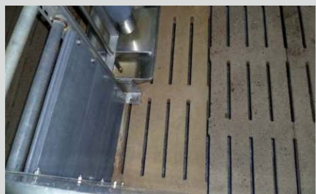
Treated split tiles after several years of usage
